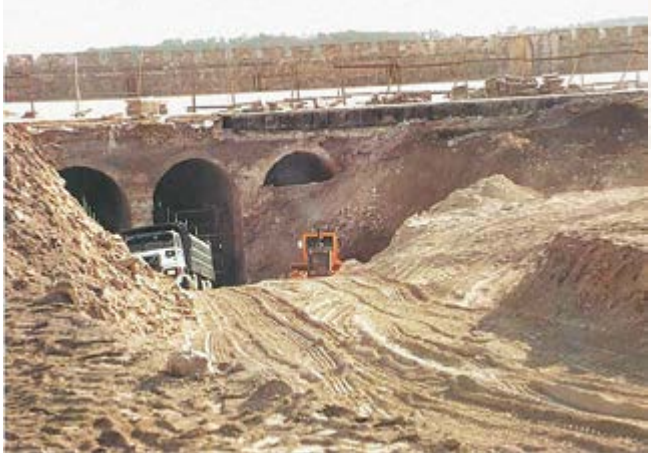
Heavy machinery used for digging a new entrance to “Solomon’s Stables” (November 1999). This work was done without archaeological supervision, removing 9,000 tons of earth, rich with ancient artifacts.
